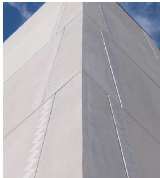
Horizontal ribbons of white tile are embedded in the concrete surfaces of the pylons to emphasise the inclined plane.
